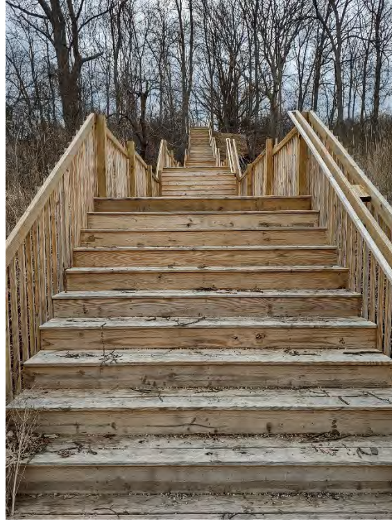
Photo 2 facing north: visible shifting of boardwalk section.
