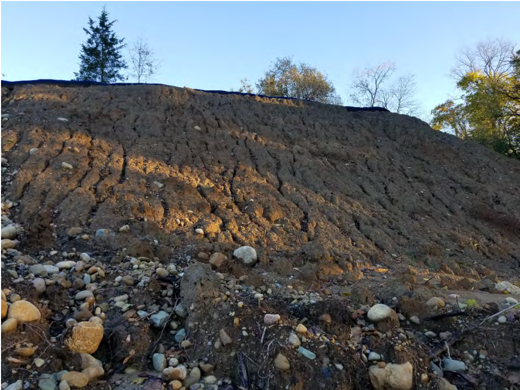
Photo 2: Erosion along slope (typical)
