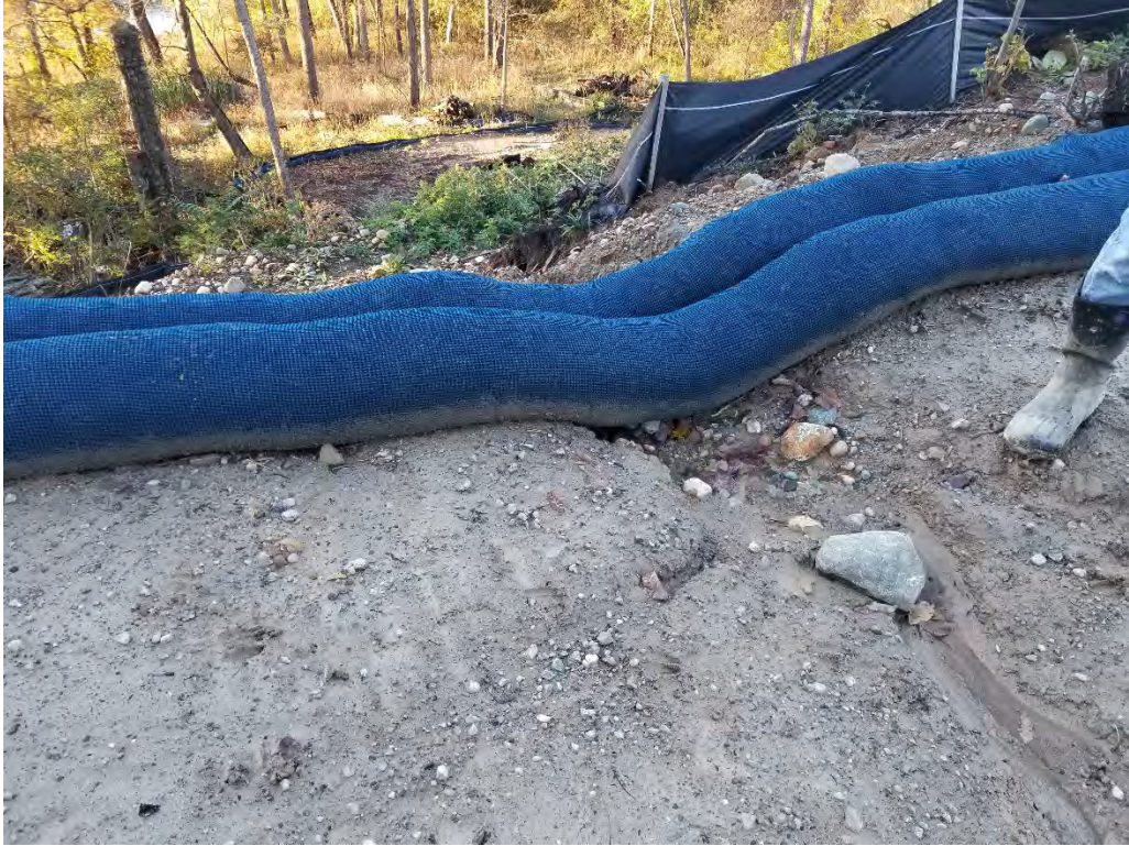
Photo 4: Runoff undercutting silt fencing
