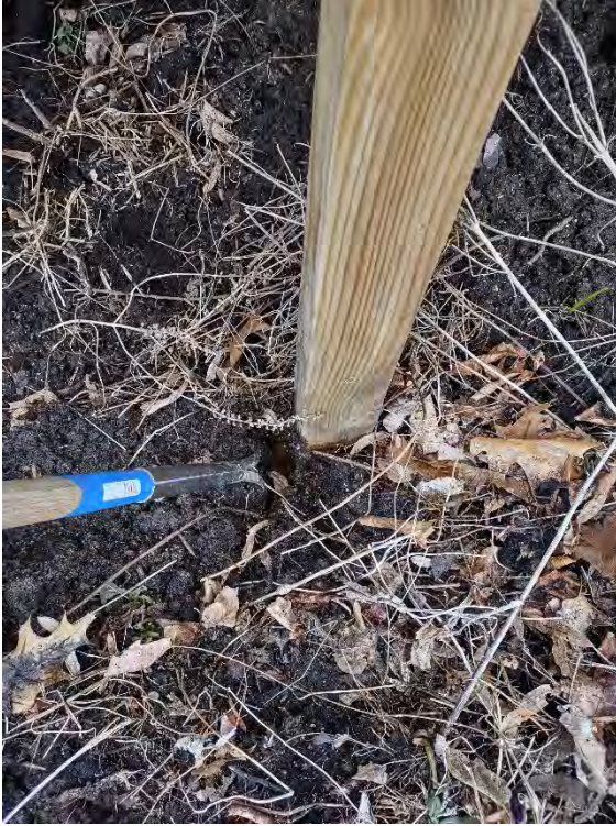
Photo 1: boardwalk posts installed directly into wetland soil without concrete foundations.
