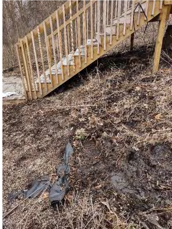
Photo 5 facing west: pea gravel over geotechnical fabric within wetland, to the east of boardwalk.
