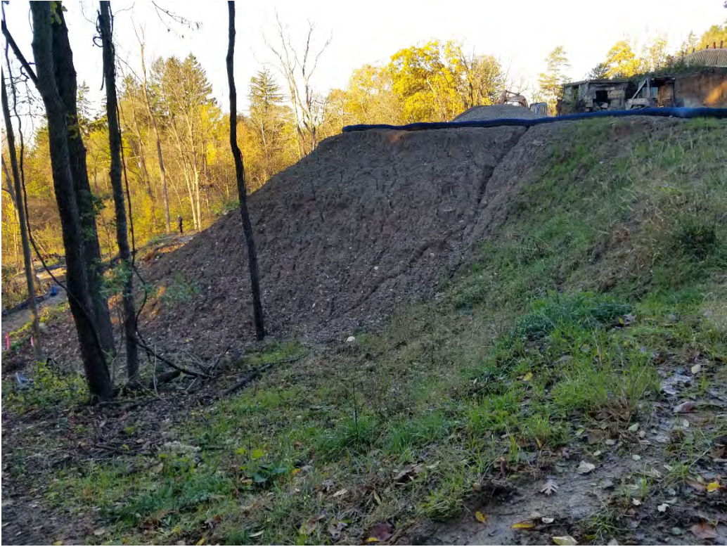
Photo 3: Erosion along slope
