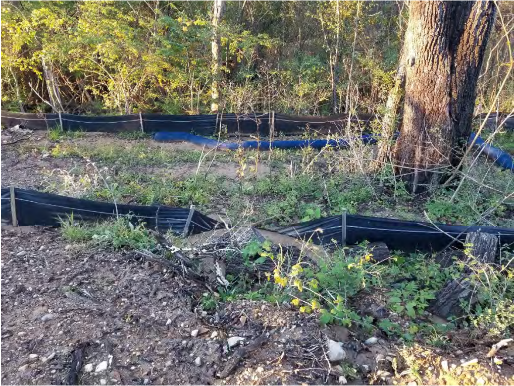
Photo 1: Silt fence failure at bottom of slope
