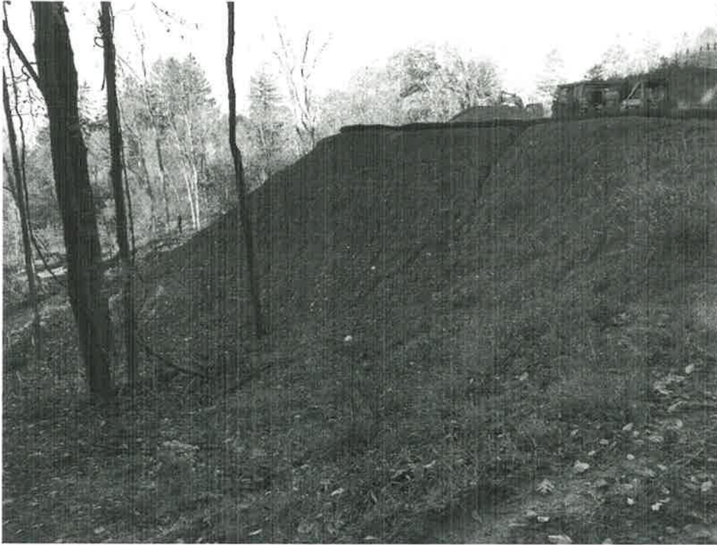
Photo 3: Erosion along slope
