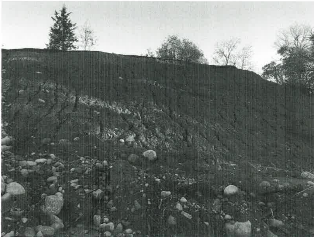
Photo 2: Erosion along slope (typical)
