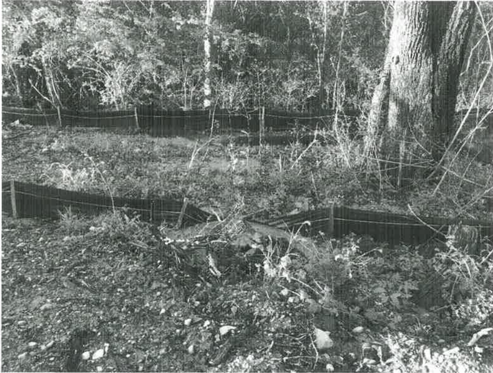
Photo 1: Silt fence failure at bottom of slope
