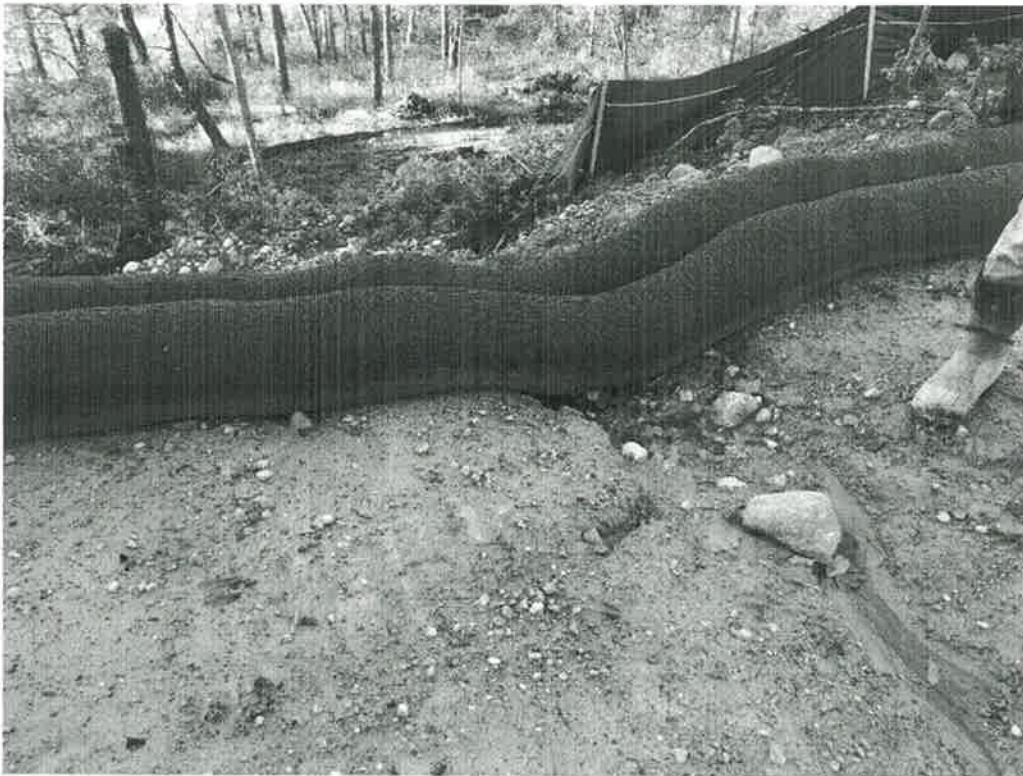
Photo 4: Runoff undercutting silt fencing
