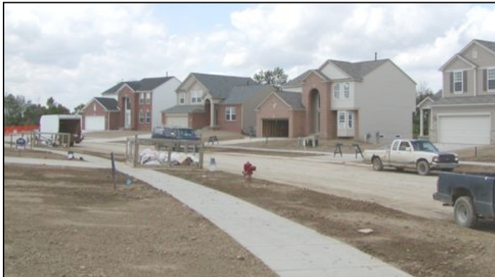
Photo 4-12: Sanitary sewer and water service is provided to new houses south of Geddes Road.
