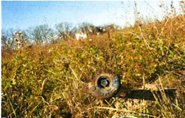
A water tap in the Lincoln Pines subdivision is shown.
