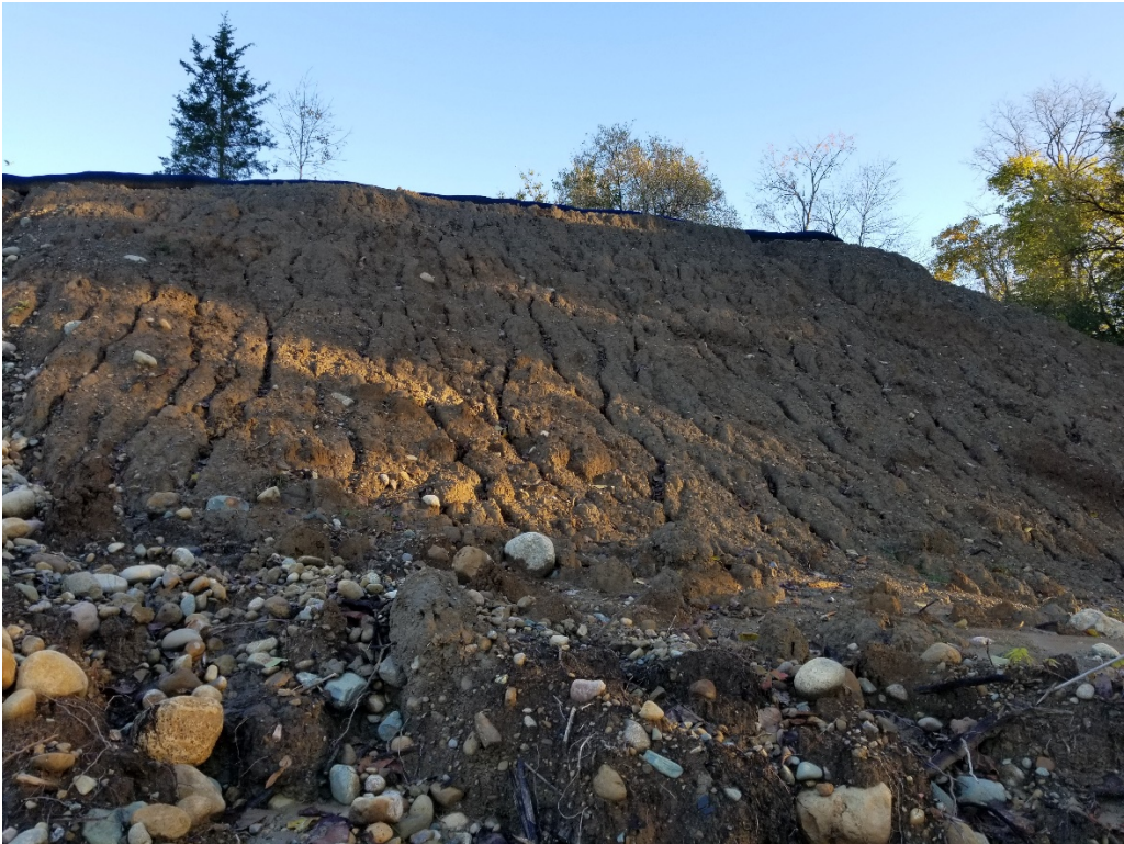
Photo 2: Erosion along slope (typical)
