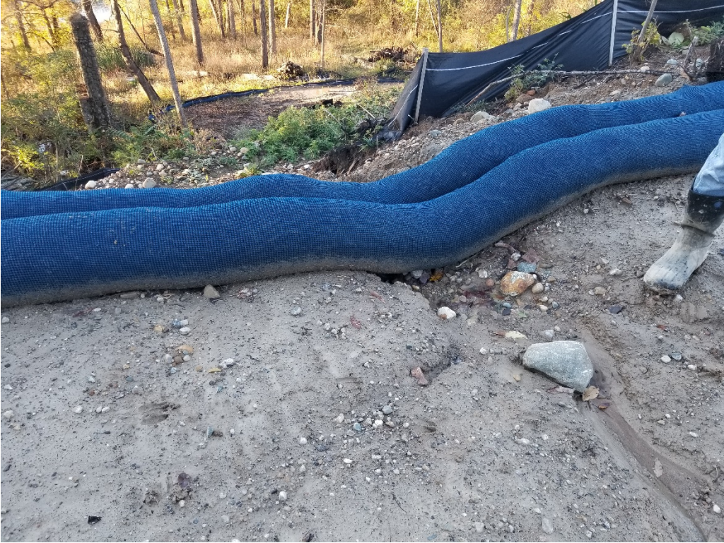
Photo 4: Runoff undercutting silt fencing
