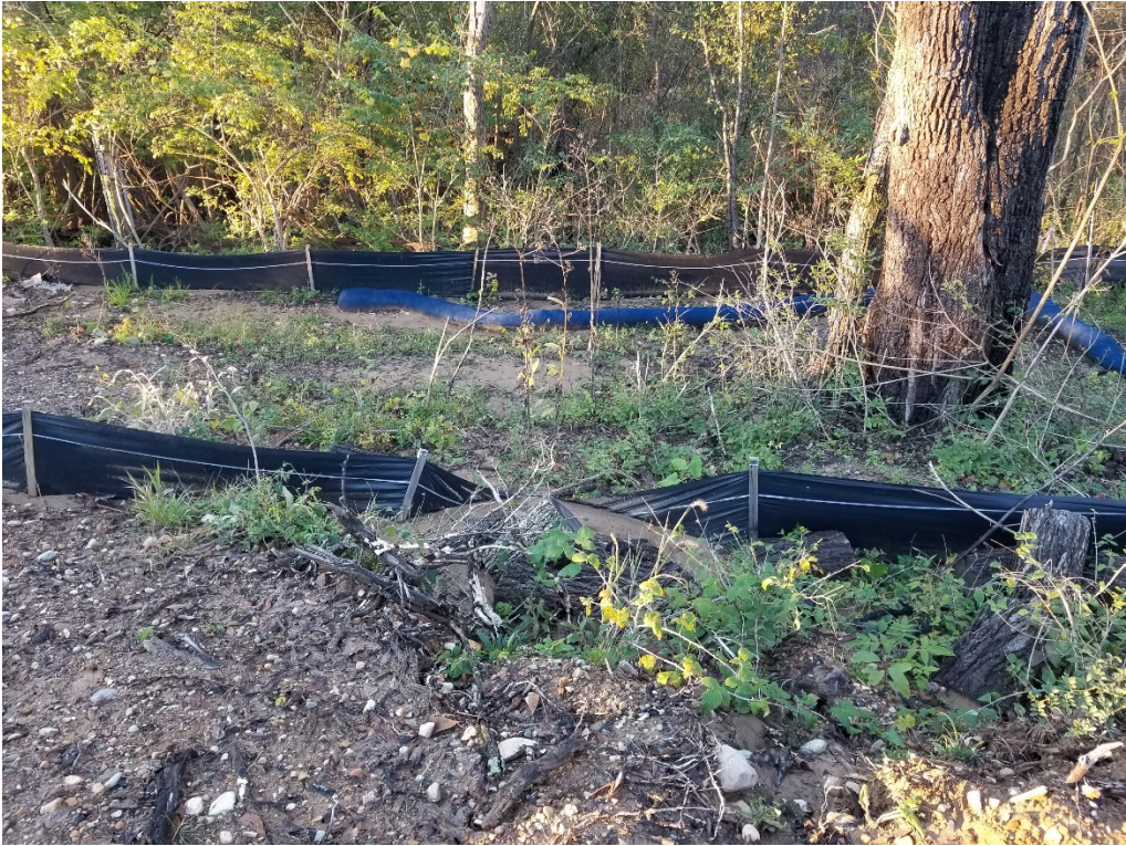
Photo 1: Silt fence failure at bottom of slope
