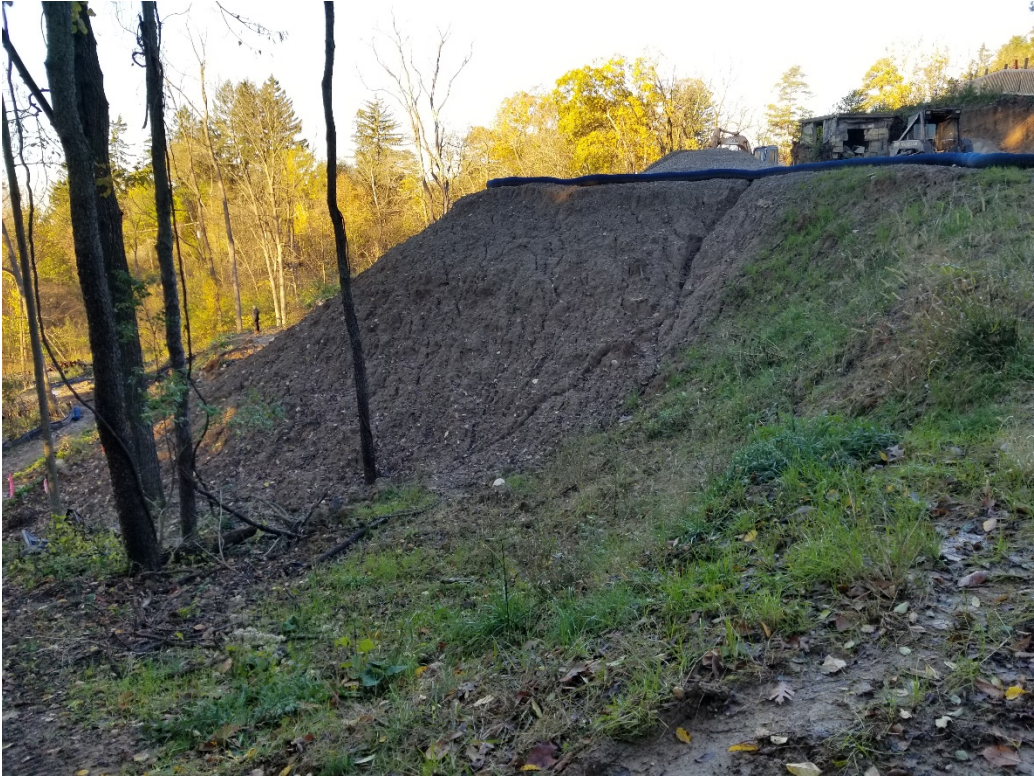
Photo 3: Erosion along slope
