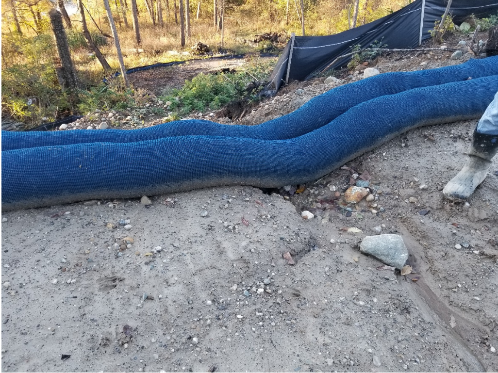
Photo 4: Runoff undercutting silt fencing
