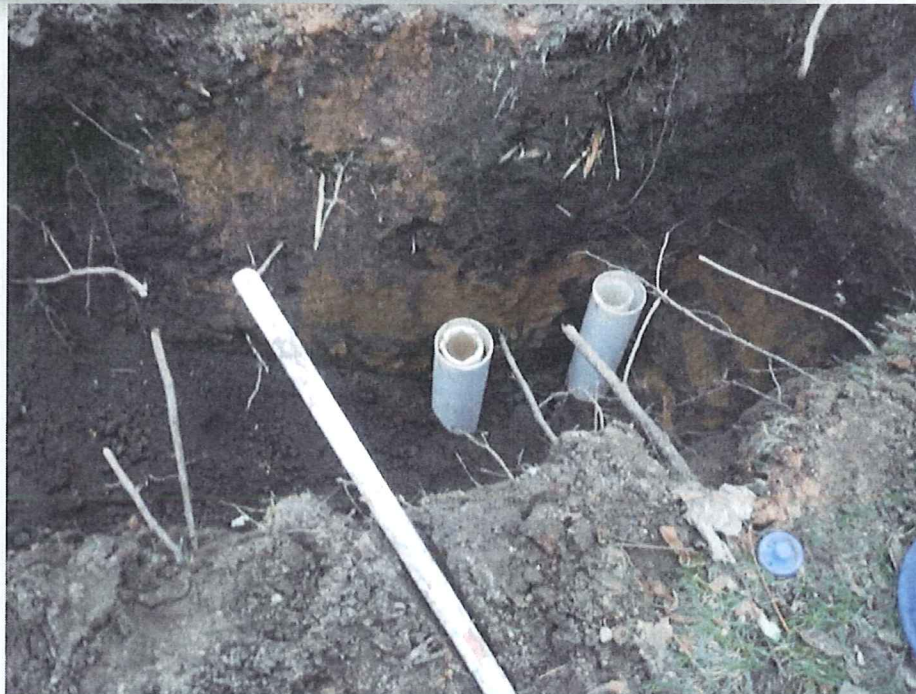
Photographs of Test Pit No. TP-3 (Top) and Test Pit No. TP-4 (Bottom) 11-16-2017
